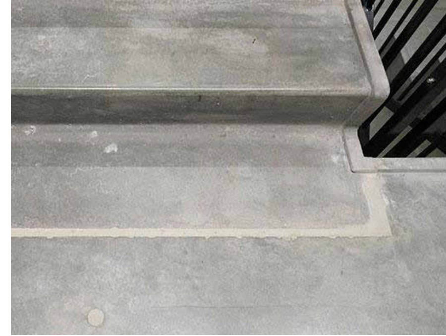
CONCRETE JOINT Joint between stairwell and landing made in the same concrete corresponding to the elements. The joint must be cast on the construction site after assembly. The cast assembly will not be able to be fully hidden.
